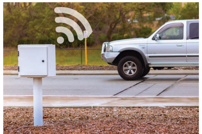
The roadside cabinet includes a solar panel, back up battery & modem that securely transmits data remotely.
