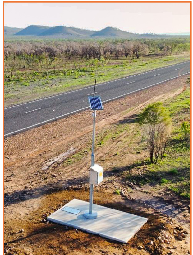
Client supplied solar panel and cabinet housing the RTG
