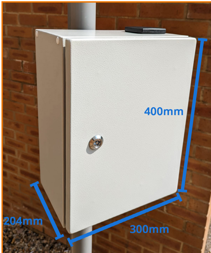
MetroCount pole mounted cabinet
